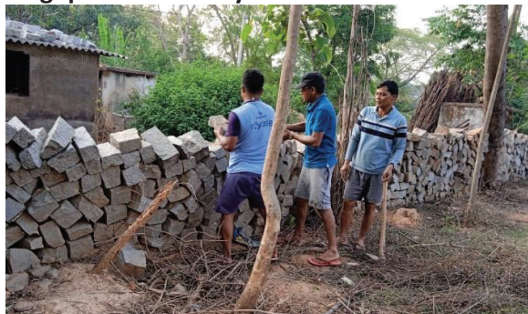
Brothers join hands and hearts as they collaborate in building a community wall.
